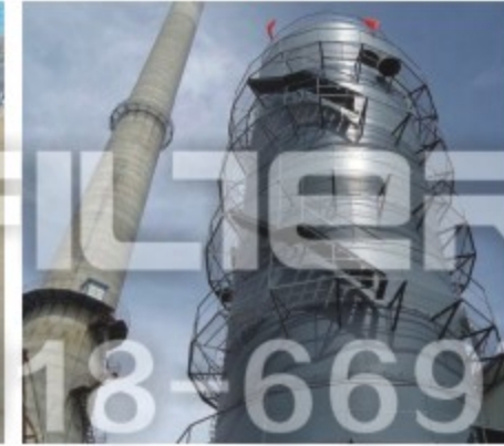
脱硫设备 The desulfurization equipment
